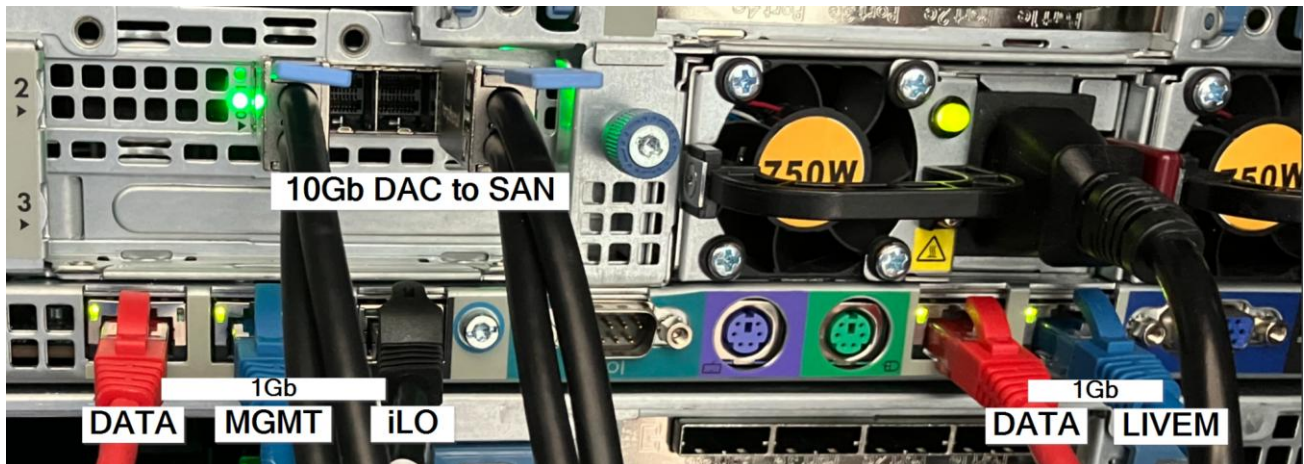
Figure 1. Rear cabling reference for the temporary hosts, showing dedicated data, management and live-migration connections alongside 10Gb DAC SAN connectivity.
